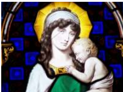
Caritas panel – window in S. Aisle(cracked)
